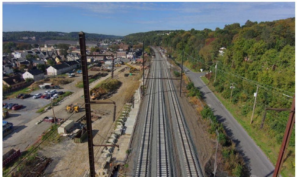
Coatesville Station during construction Copyright Commonwealth of Pennsylvania Department of Transportation, 2024. All Rights Reserved. Used by Permission
