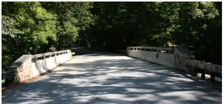
Park Lane Bridge over East Branch of Brandywine Creek in Glenmoore, Wallace Township.
